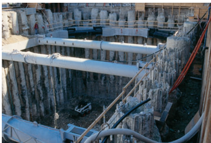
Photo 6 Station de Christianshavn. Butonnage en tête de fouille Christianshavn station. Bracing on excavation head
