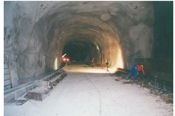
Photo 3 Intérieur du tunnel (pose des bordures) Inside of tunnel (placing of curbs)
