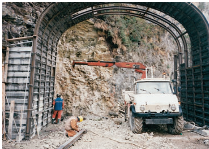
Photo 2 Tête aval du tunnel (pose de cintres) Downstream head of tunnel (placing of arches)
