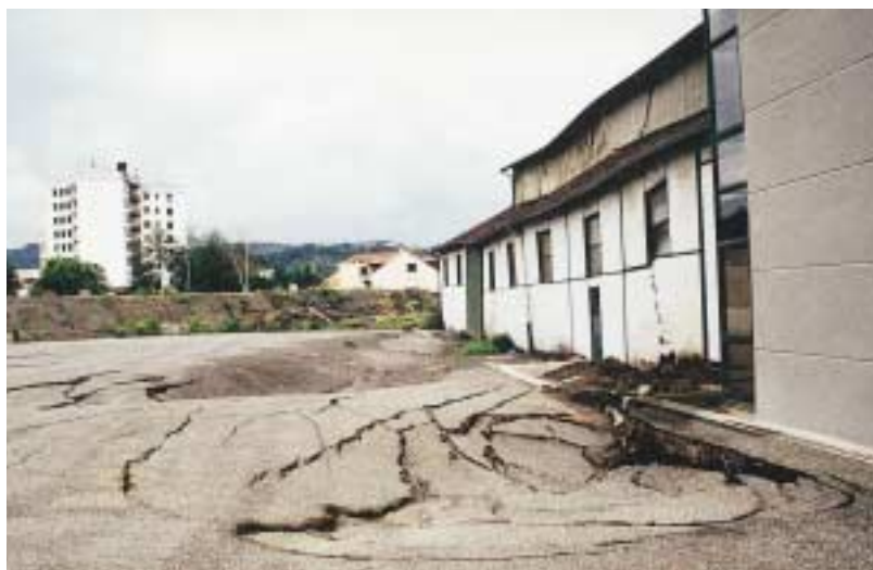
Photo 1 Bâtiment Transville : crevasses et affaissements de la chaussée, bâtiment endommagé. Arrière-plan : remblai houiller Transville building: cracks and sinking of pavement, with damage to building. Background: coal-field embankment
