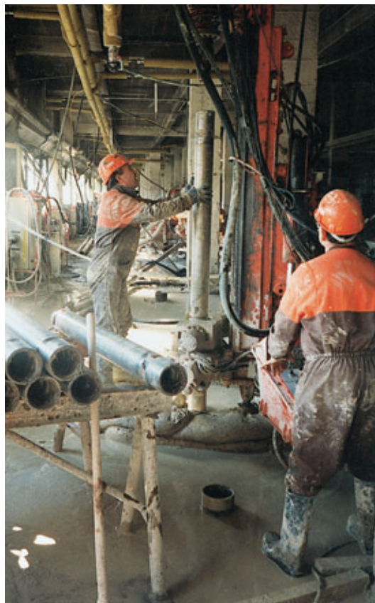
Photo 2 Foreuse Soil Mec 350 en espace exigu Soil Mec 350 drilling rig in confined space
