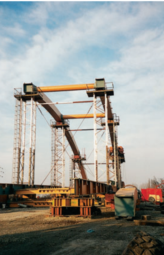
Photo 3 Assemblage de l'ouvrage rive sud Assembly of the structure on the south bank
