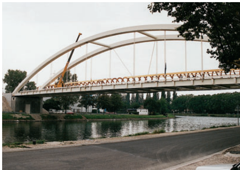
Photo 2 L'ouvrage en place. Le passage piétons et cycles en cours de montage The structure in place. Pedestrian and cycle paths being completed
